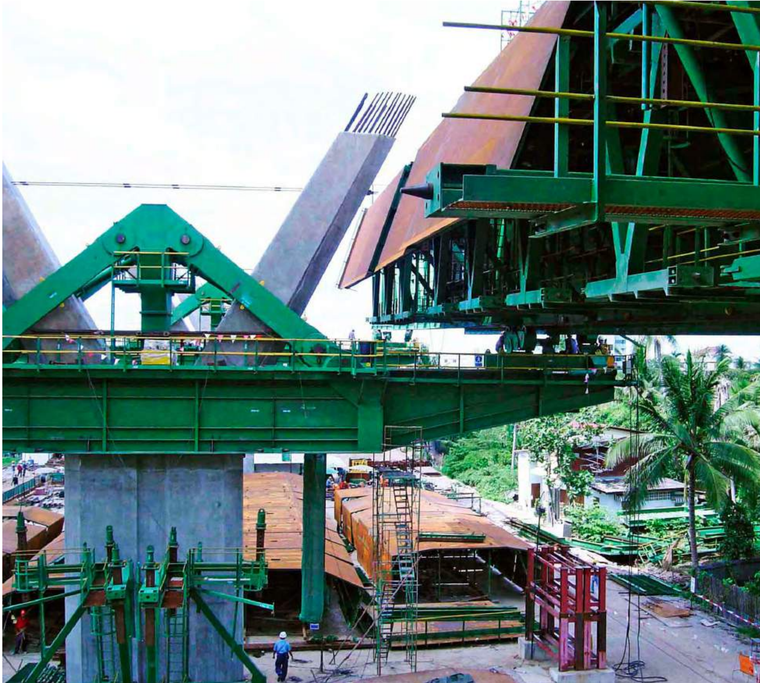
Underslung MSS with steel formwork and launching wagons with wheels – Industrial Ring Road, Thailand
