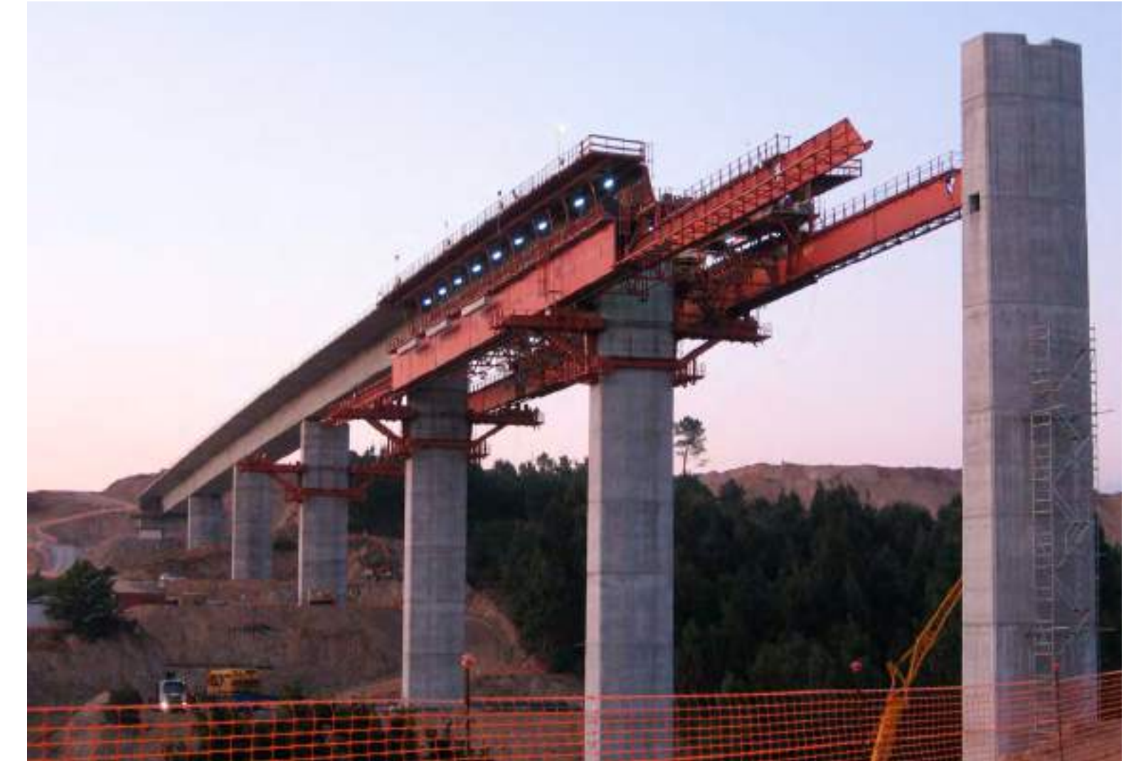
Supporting brackets supported on the column and blockout visible in the front column
