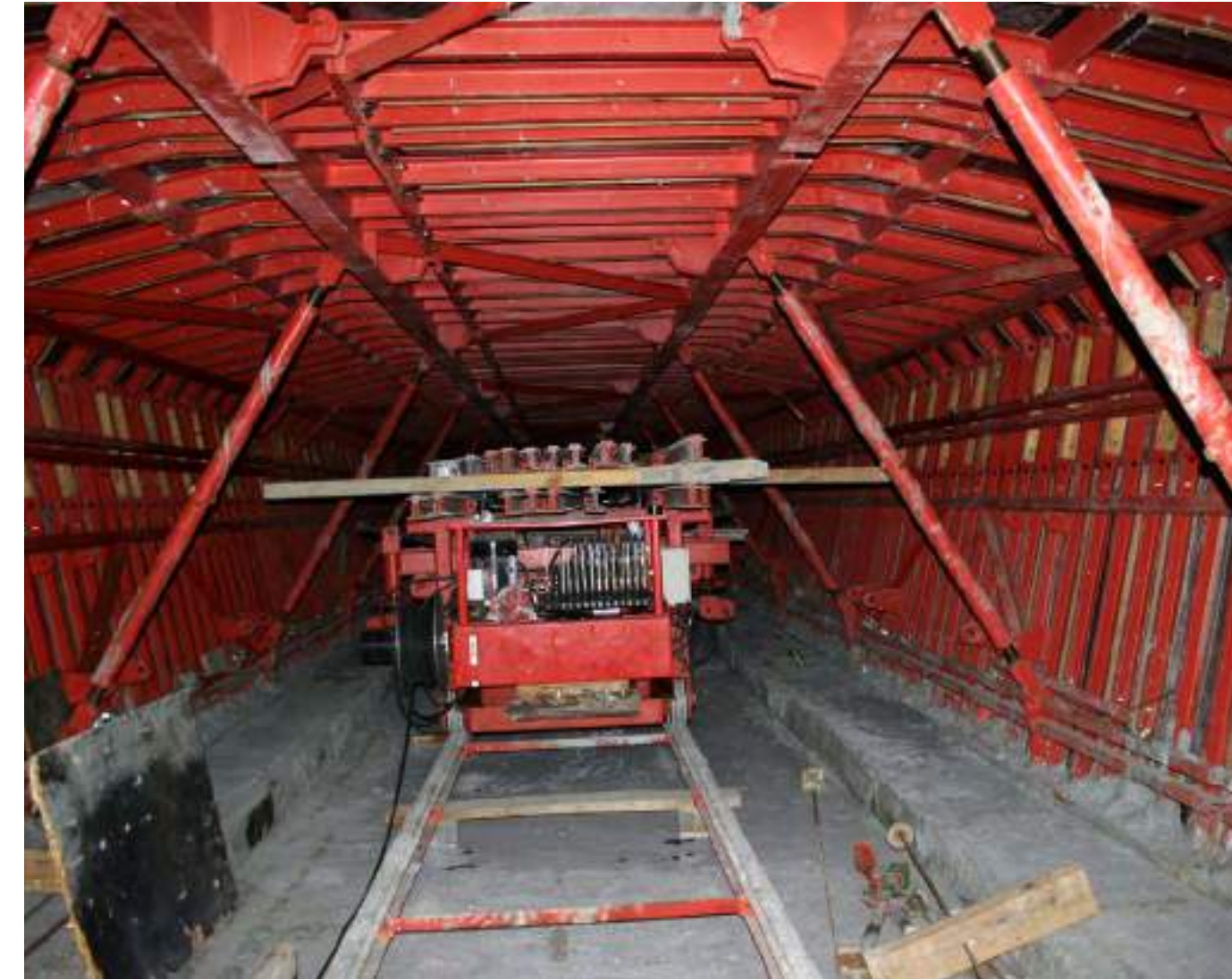
Use of the transport trolley to relocate the rails on the next span
