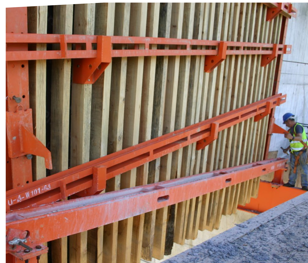
External formwork– vertical saw wooden beams and horizontal steel beams acting as strongbacks
