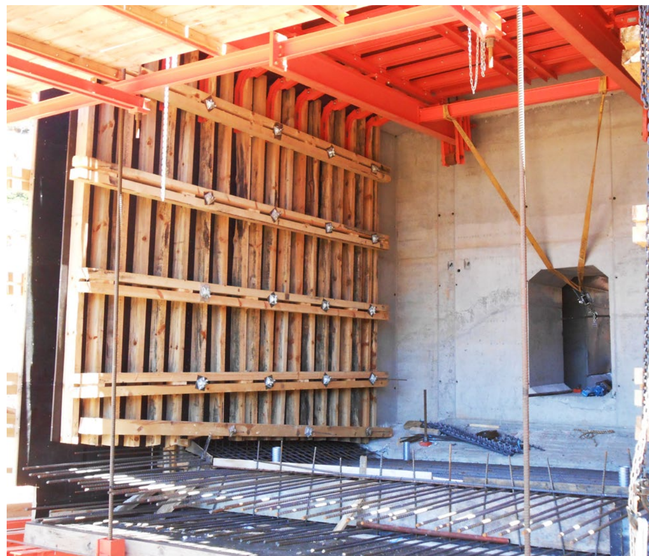
Internal formwork – vertical saw wooden beams and horizontal saw wooden beams acting as strongbacks
